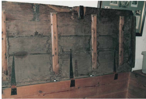
Fig. 16 'Bites' showing two of original four positions of mortised knuckle hinges, Faversham.
